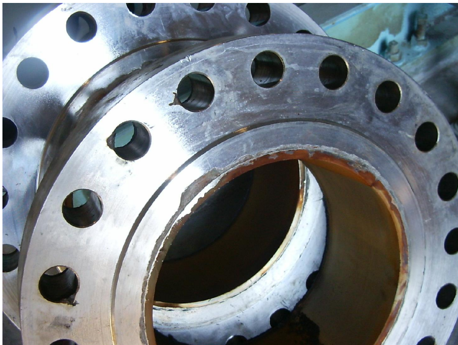
FIGURE 6 - Corrosion of a superduplex flange with a PTFE coated gasket.
